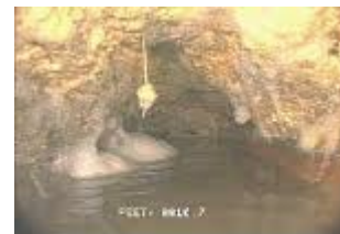
Grease on walls of a sewer pipe
